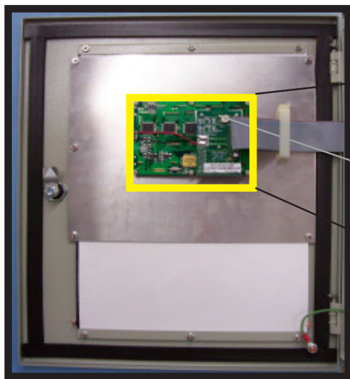
Back of door showing the LCD Display Board
