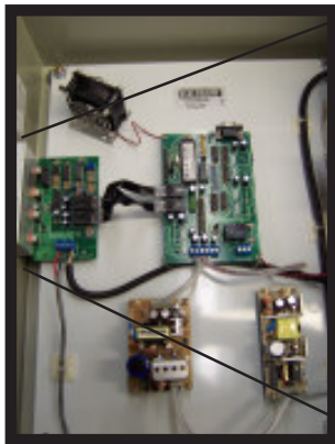
View showing all boards.
