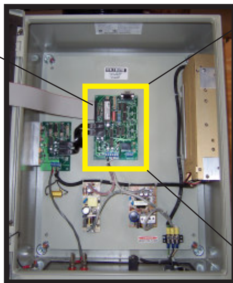
View of Main Control PC Board
