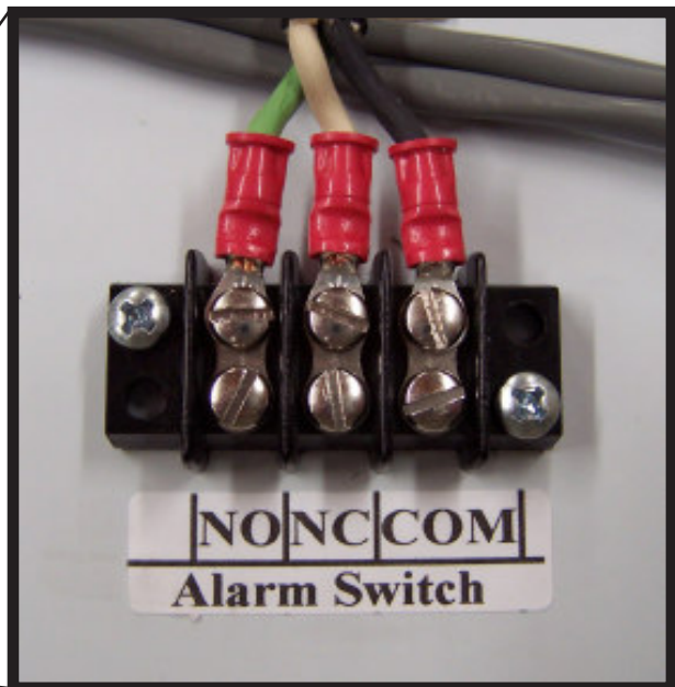
Close-up view of Terminal Strip
