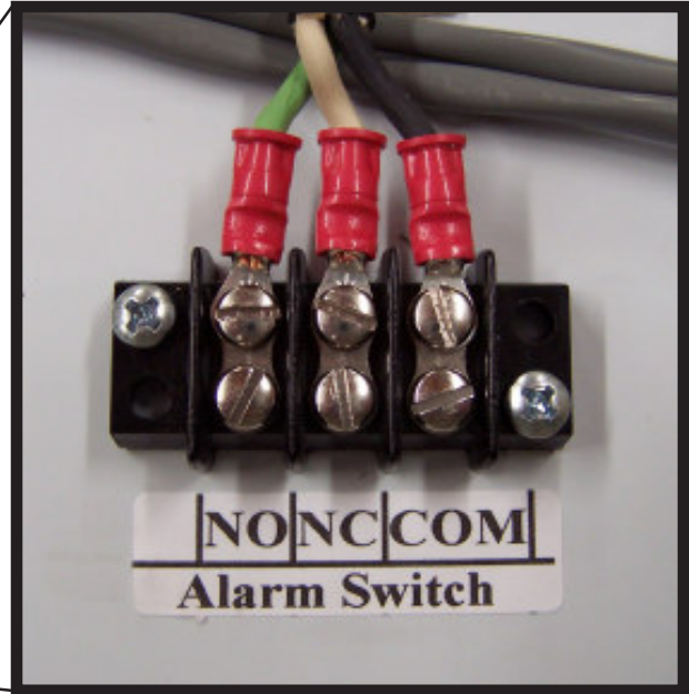
Close-up view of Terminal Strip
